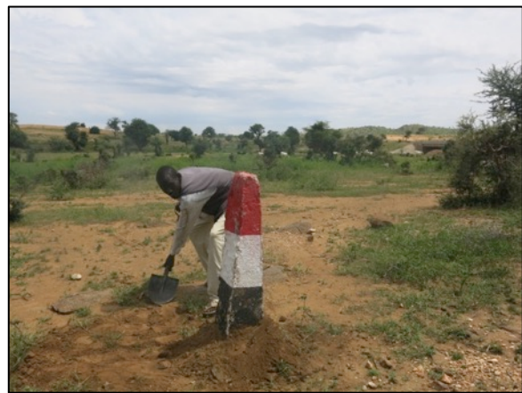
Installation of the fabricated edge markers in Sornei village close to Zalingei.
